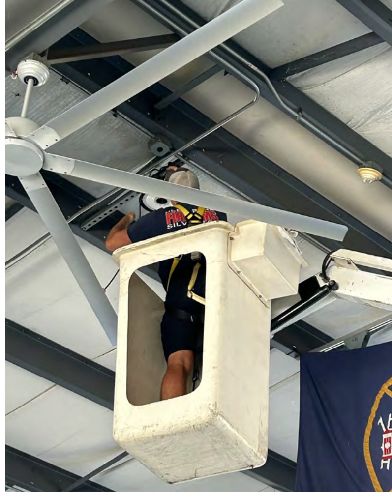
Firefighter/EMT Mark Landesman replaced outdated bay lighting with new energy-efficient LED lights during routine station maintenance on August 30.
